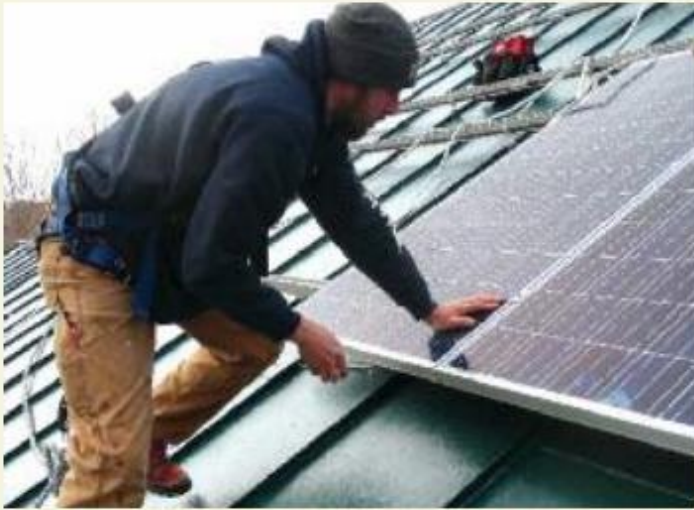
An Insource Renewables crew installs rooftop solar panels. The business is in the process of converting to a worker-owned co-op. Photo courtesy Insource Renewables
