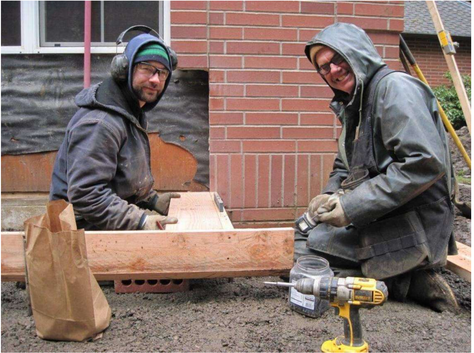
A-1 Builders employees Justin Deane and Mike Gill are at work preparing a brick wall for a new door. A-1 Builders will become a worker-owned cooperative in July. A-1 Builders - Courtesy to The Bellingham Herald
